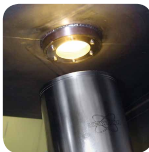
Connecting the sensor head to a viewing window of a reactor.
